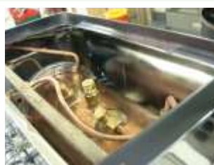
Inside the machine. Note the new safety valve.
