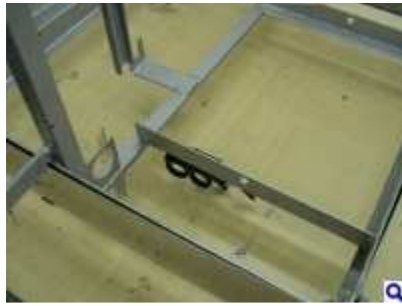
Frame with the electrical cable strain reliefs installed.
